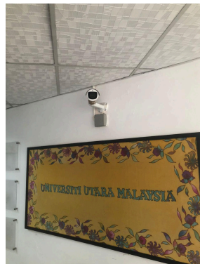
Figure 4: The CCTV facing class halls
